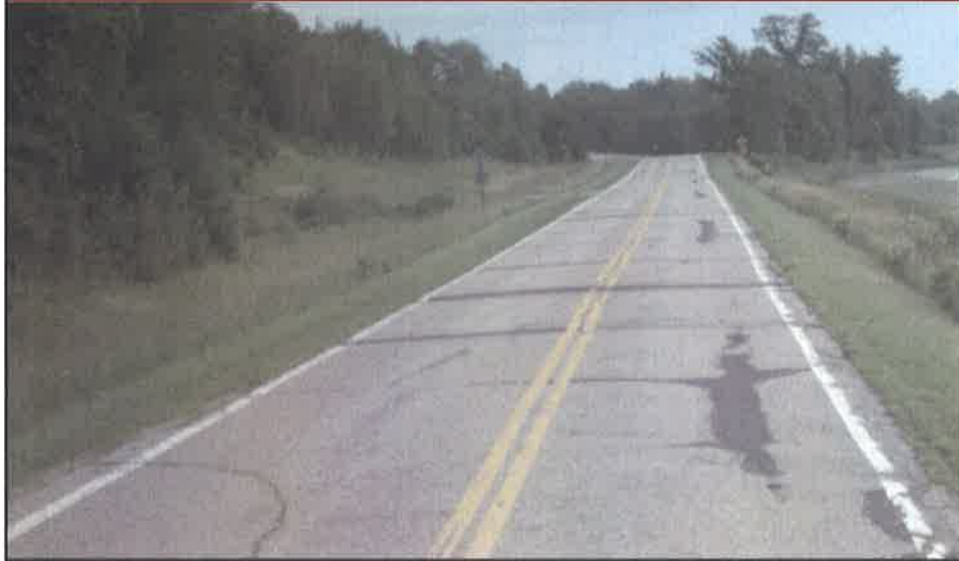
Example road conditions PQI = 1.9
