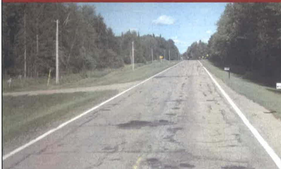
Example road conditions PQI = 1.3
